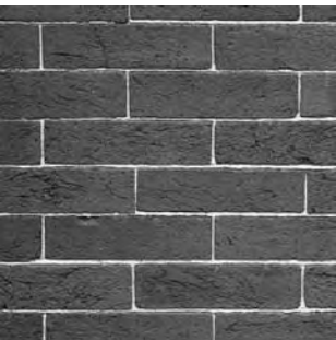
19th C. ground face brick common bond, narrow mortar joints Worcester County Courthouse photo Karen Houtman
