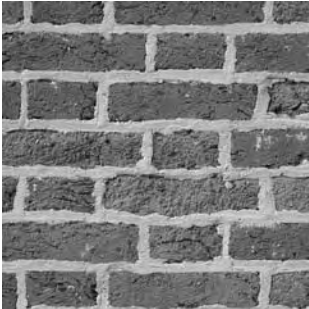
18th C. soft brick Flemish bond, badly repointed
