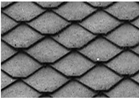
above: "Transite" asbestos roof. Because the asbestos fibers in "transite" are embedded in a solid medium, they are not readily released into the air as would occur if the material was cut or abraded with a power saw or sander. Therefore, transite is not regarded as a significant health hazard. Asbestos roofs are not an environmental hazard unless they are broken or crumbled and the dust inhaled. That is why, when removed, they fall under the hazardous materials regulations. If left in place, they make a good roof.
