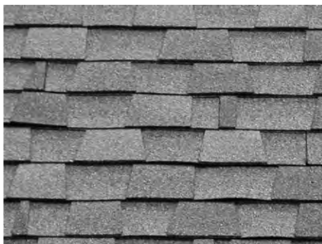
below: Asphalt shingles have become the most common roofing material in the present time. While relatively inexpensive, their life expectancy cannot compare with slate or standing seam metal.
