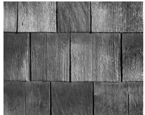
above: Wood shingles are a traditional roofing material on the Eastern Shore. Some early ones were made from Cypress but these are no longer available. In the colonial era, the shingles were nailed to laths, which were nailed to roof rafters. They were visible from the attic below and air could circulate. Some of the early roofs lasted over 100 years. Present day shingles made from Cedar can be very durable, especially if installed in a way that allows them to breathe.
