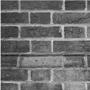
18th - early 19th C. soft brick incised mortar joint. The molding is called a water table.
